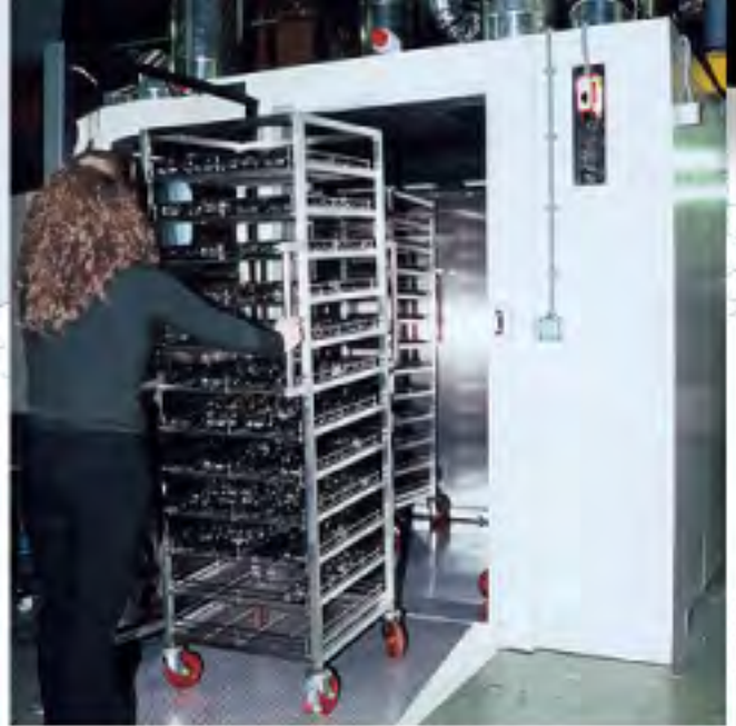
Steady state, high temperature room with clean filtered air cooling. Designed for heat conditioning automotive electronic components as part of a high volume production process.
